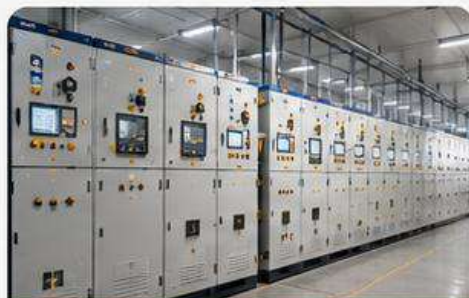
Electrical Power Systems
